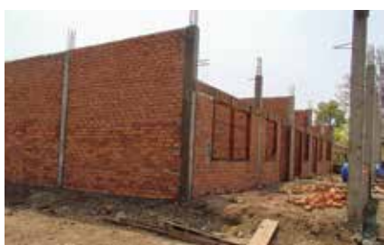
The design of this under construction preschool in Cambodia took Villanova's Engineering team to the SEI Student Structural Design Competition finals.
